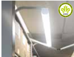
AUTOMATIC OVERHEAD AISLE LIGHTING
